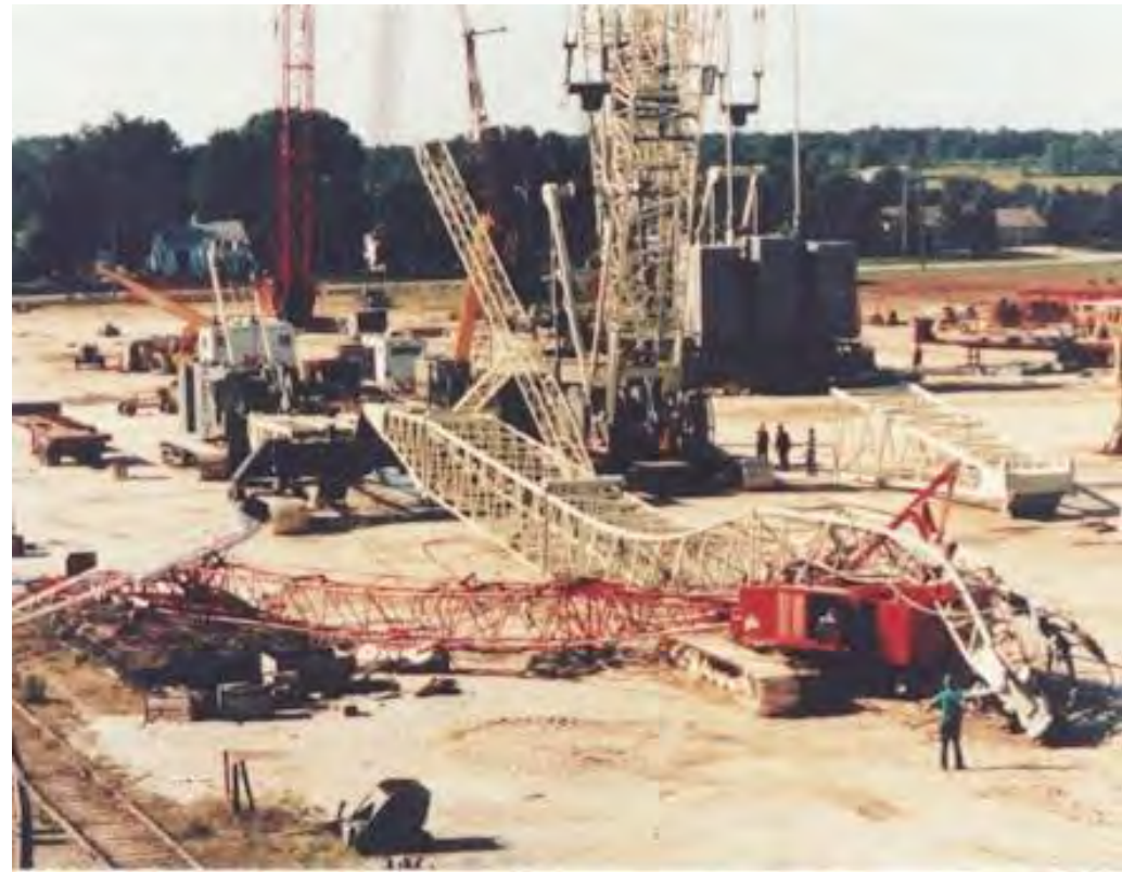
Picture 2: Crawler crane after breakage of the suspension rope
