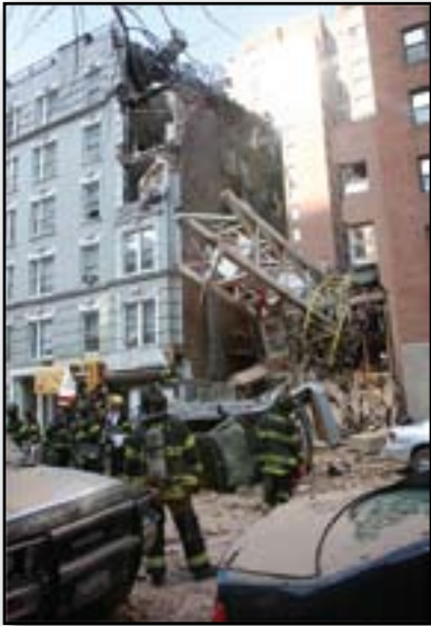
Chang W. Lee/The New York Times The scene of the fatal collapse of a 22-story crane on Manhattan's East Side in March.
